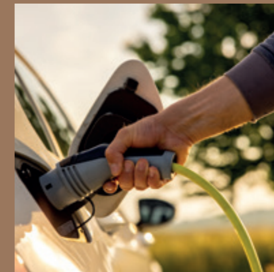
Electric car charging stations
